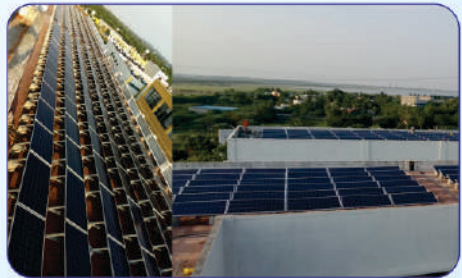
CIT CHENNAI, SOLAR PROJECT 300KWP
